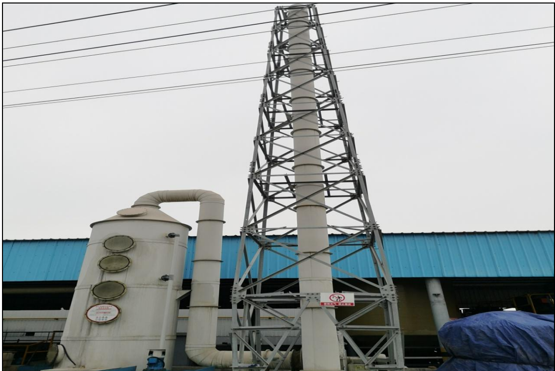
絮凝剂生产线、乏酸储存、盐酸储罐、危废库废气排气筒及废气处理设施
