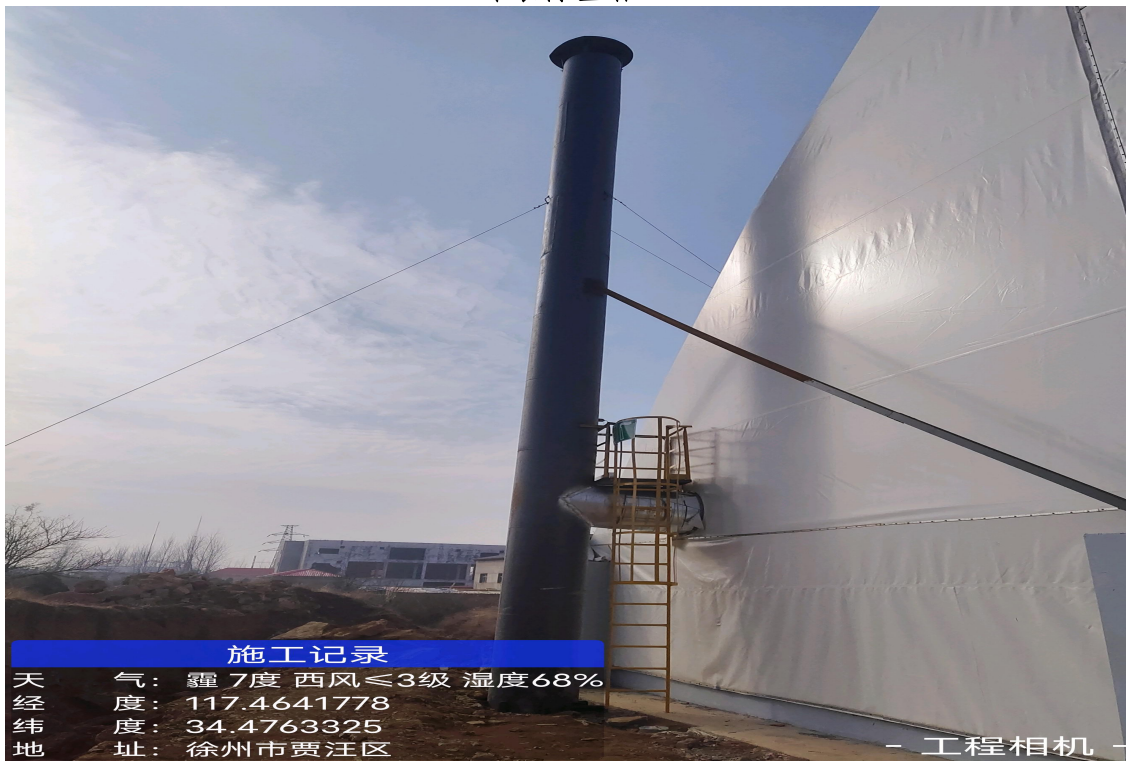
1#暂存库废气排气筒
